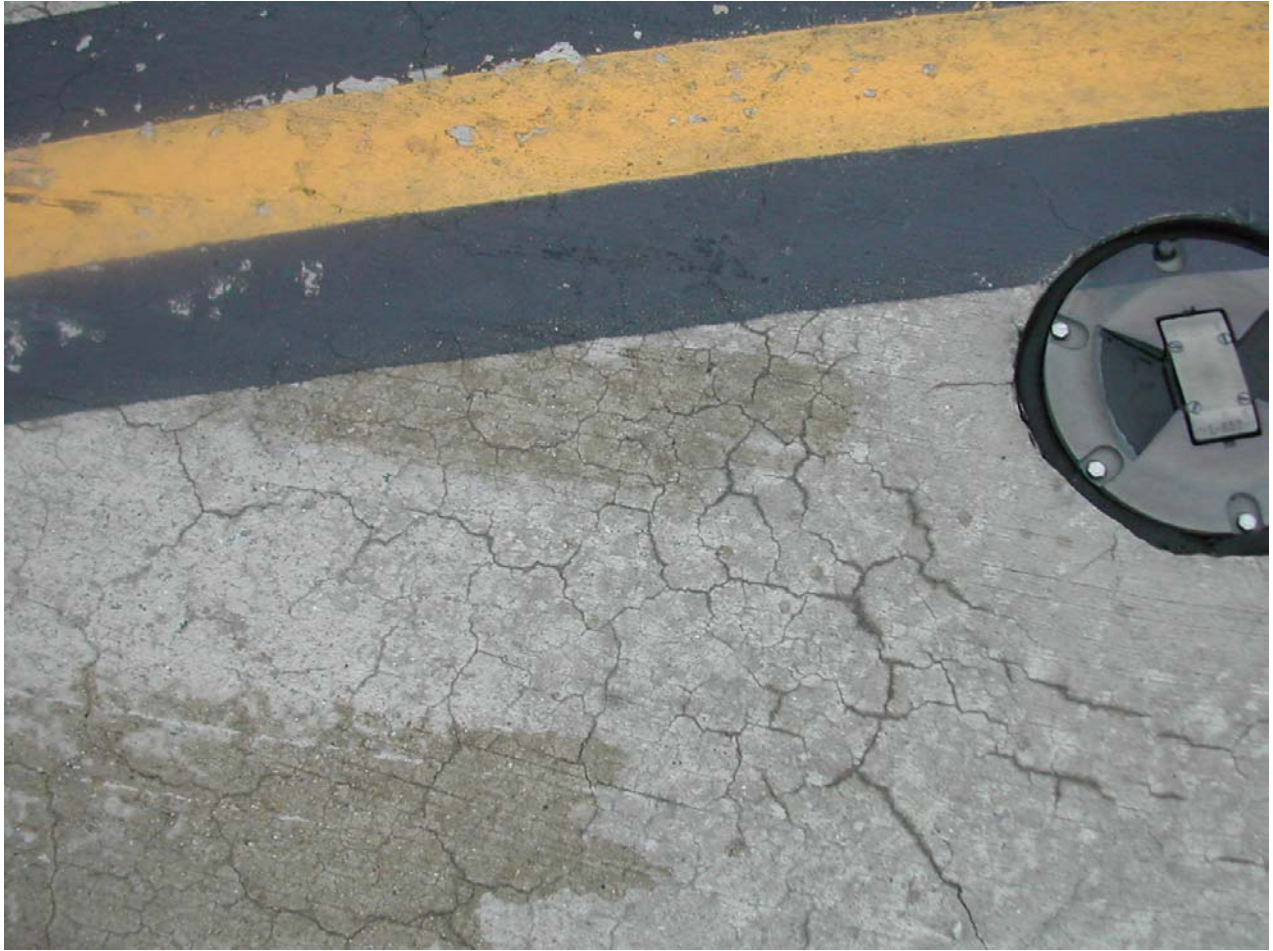
FIGURE 1. TYPICAL DISTRESS OBSERVED IN CONCRETE PAVEMENT EXPOSED TO AIRFIELD DEICING CHEMICALS
